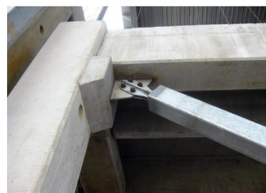
Typical upper connection of buckling-restrained brace to precast concrete beam and column.
